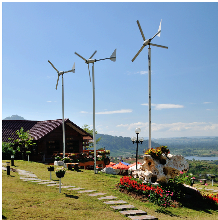
Home equipped with a wind power system converting wind into electricity.
